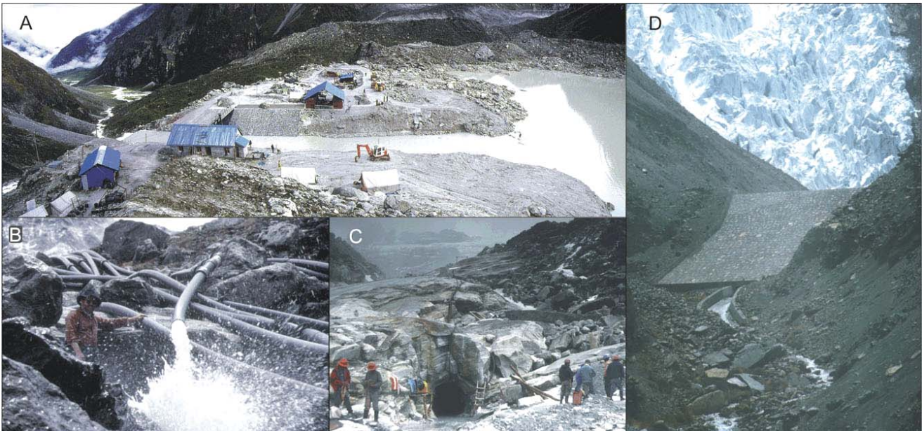
Fig. 15: Examples of glacial lake hazard remediation styles. A - channel with control gates, Tsho Rolpa, Nepal; B - Siphons, Tsho Rolpa, Nepal; C - tunnel through bedrock cored moraine dam, Lake 513, Peru; D - channel and reconstructed dam, Cuchillacocho, Peru (photo César Portocarrero).
